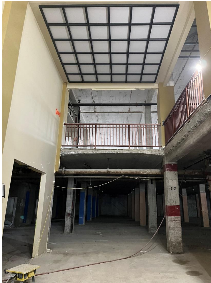
Photo 10. First floor, original 1911 building, contemporary entry lobby area at south side of the floor with partially removed contemporary office finishes, view north.
