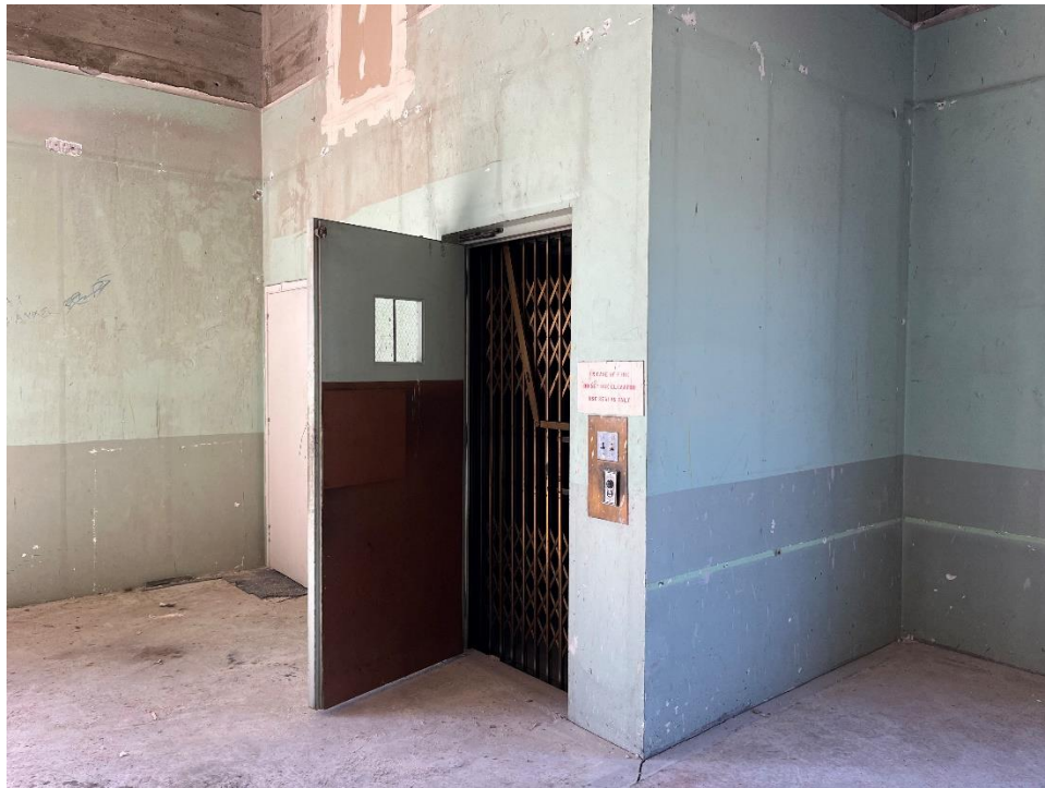
Photo 24. Fourth floor, 1947 addition, passenger elevator, view northwest.
