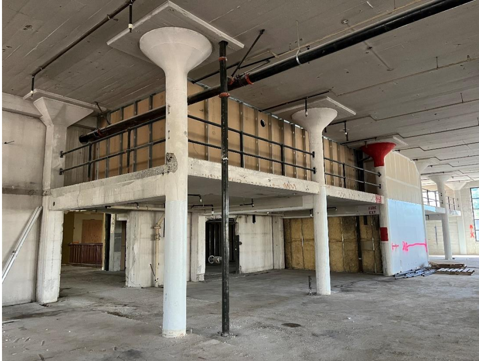
Photo 17. Second floor, 1936 west addition, concrete mezzanine and freight elevator enclosure, view southeast.
